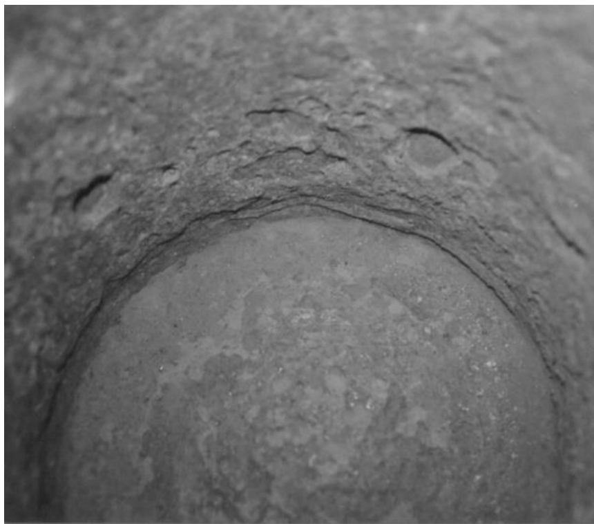
Figure 15: Corrosion at the bottom of a condemned carbon dioxide cylinder
