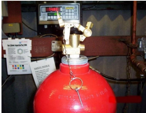
Figure 14: Quick opening cylinder valve for fire suppression system with locking device disengaged and valve open
