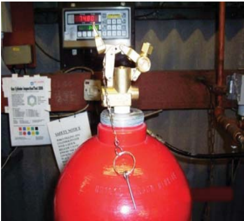
Figure 15: Quick opening cylinder valve for fire suppression system withlocking device disengaged and valve open
